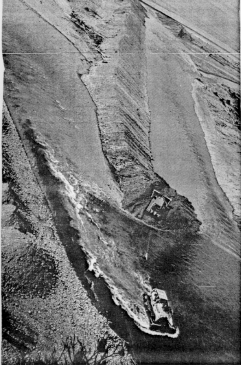
MOVING A RIVER — A bulldozer crosses the old channel after cutting through the last of gravel Thursday to allow the Elwha River to turn into a new channel at its mouth. A new bed for the river was dug after it had cut its way westward to a point where it endangered several residences at The Place near the confluence of the Elwha and the Strait of Juan de Fuca. The Strait is in top of picture. (Evening News Photo.) May 15 - '64 (12)
