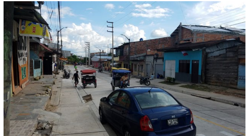
Photo by Rhiannon Neuville. A street in Iquitos with deteriorated sidewalks that pose a hazard to pedestrians.
