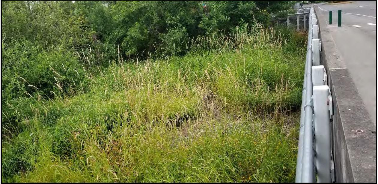
Photograph 13. South side of North Creek Parkway North bridge looking west. (T. Allard, July 2, 2019).
