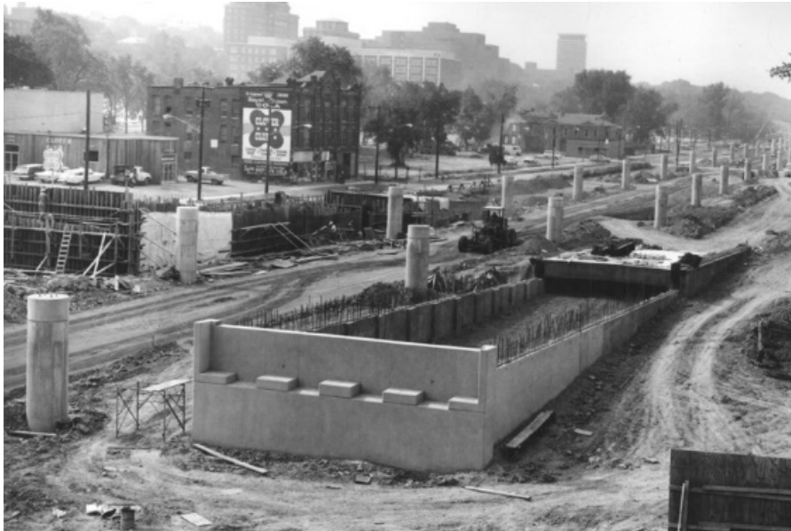
Figure 8 Construction of I-81 through the 15 th Ward, the center of Syracuse's black population in Syracuse, NY during the 1960s
