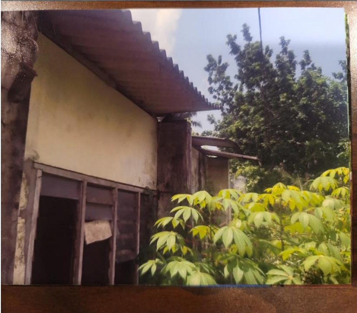
One of the many dilapidated buildings at the Uvuru Health Center
