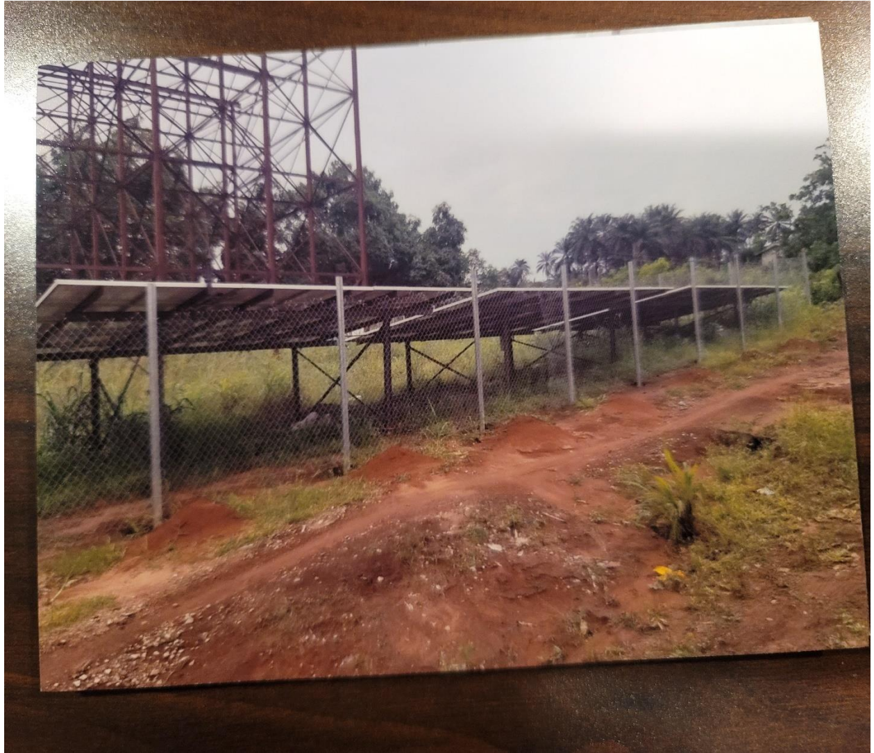
Unkempt Compound with Deteriorating Infrastructure
