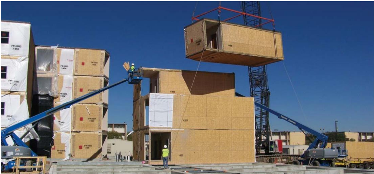
Volumetric module transportation and stacking on construction site using a tower crane (McGraw-Hill Construction, 2011)
