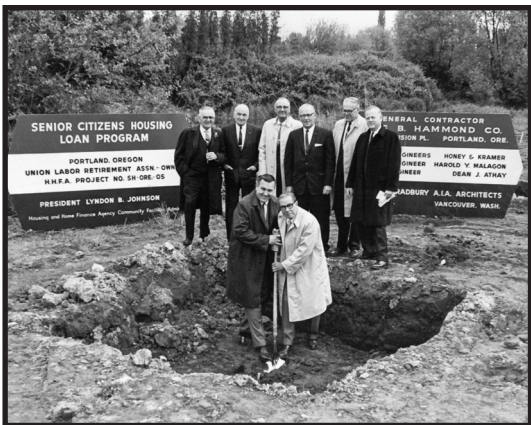
On May 3, 1965, a hole was dug marking the first stage of the $3.5 million Westmoreland Union Manor retirement apartment project.
