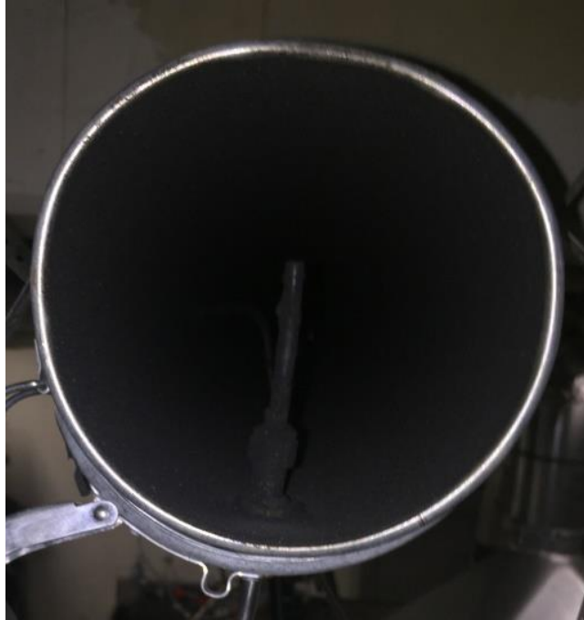
Figure 11: Sample port in the ducting. The stainless steel tubing used is inserted 3" into the ducting, and flow is drawn through to the CO/CO 2 and gravimetric filter analyzers. CO 2 samplings were performed along the duct radius at sampling locations to ensure sufficient mixing has occurred. The samplings returned a uniform CO 2 profile, suggesting that the flow is homogenous in the ducting.
