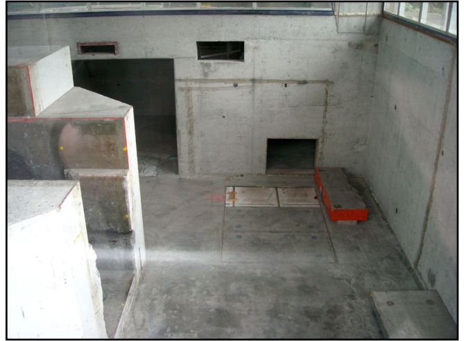
Figure 13 • Reactor room, viewing south
