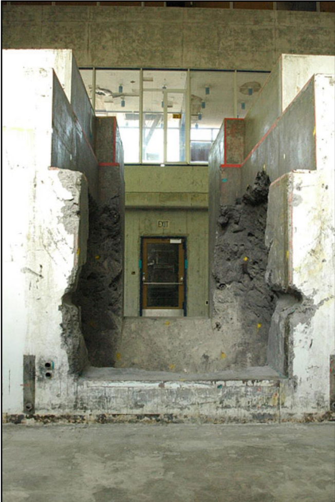
Figure 12 • Reactor room, viewing east
