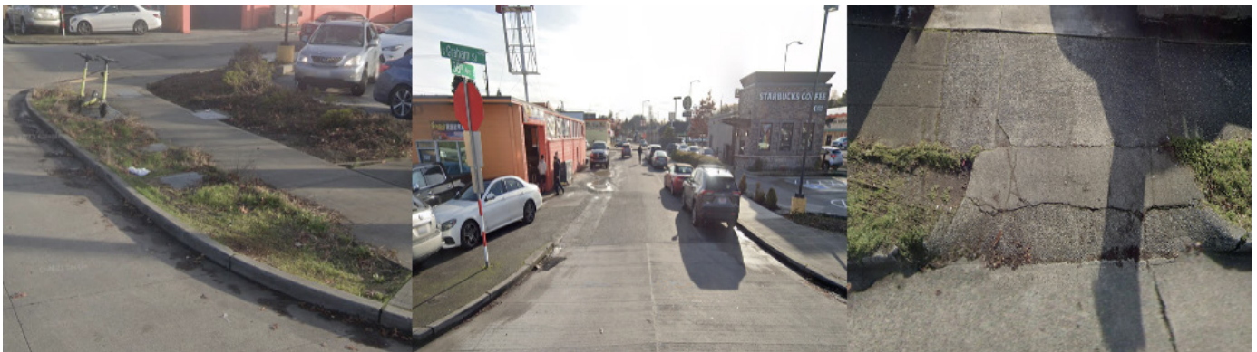
FIGURE 5-73. POOR LANDSCAPING / SIDEWALK INTERRUPTION / UNEVEN PAVEMENT
