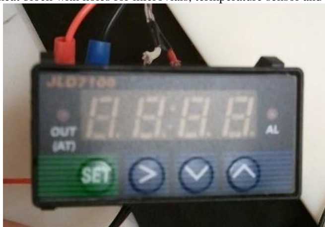
Fig. 13. PID temperature controller
