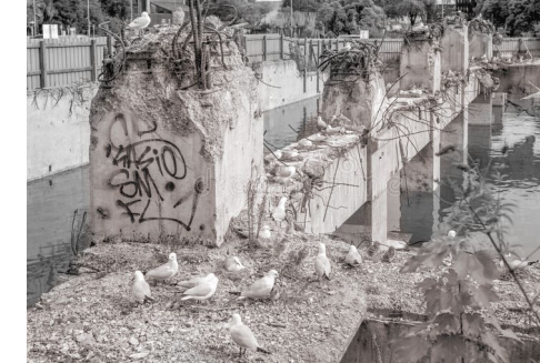
Post-earthquake: Damaged Urban Space
