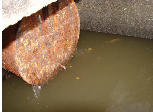
Figure 9. Rusty Backflow Pressure Lid. Michele LaFontaine
