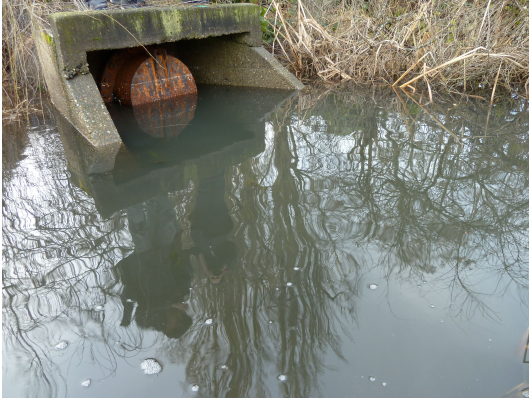
Figure 8. Holding Pond Drain Michele LaFontaine
