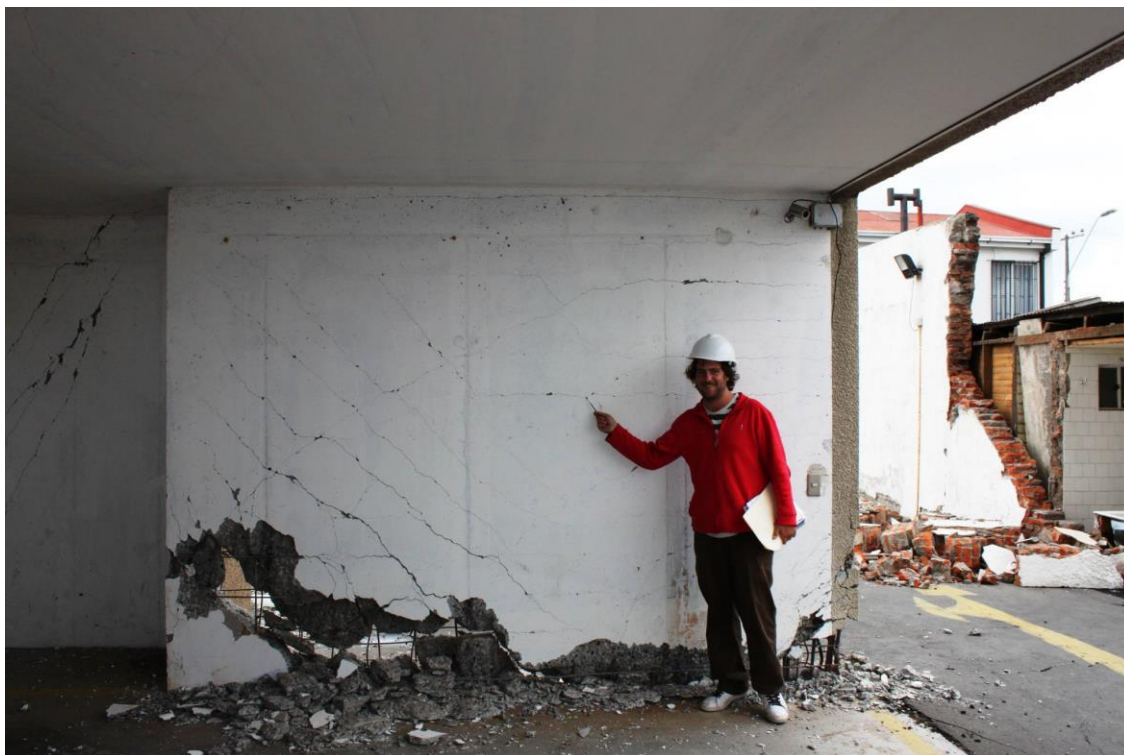
Figure 2.4 – Structural Wall Damage in 2010 Chile Earthquake (Moehle 2011)
