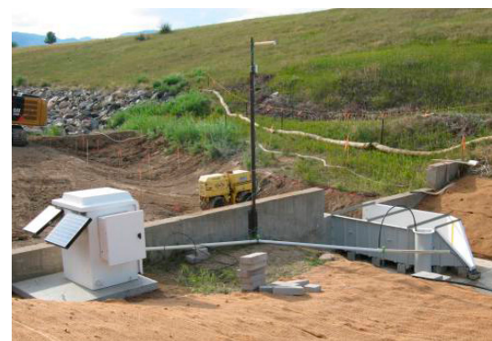
Figure 50 | Existing Monitoring Station
