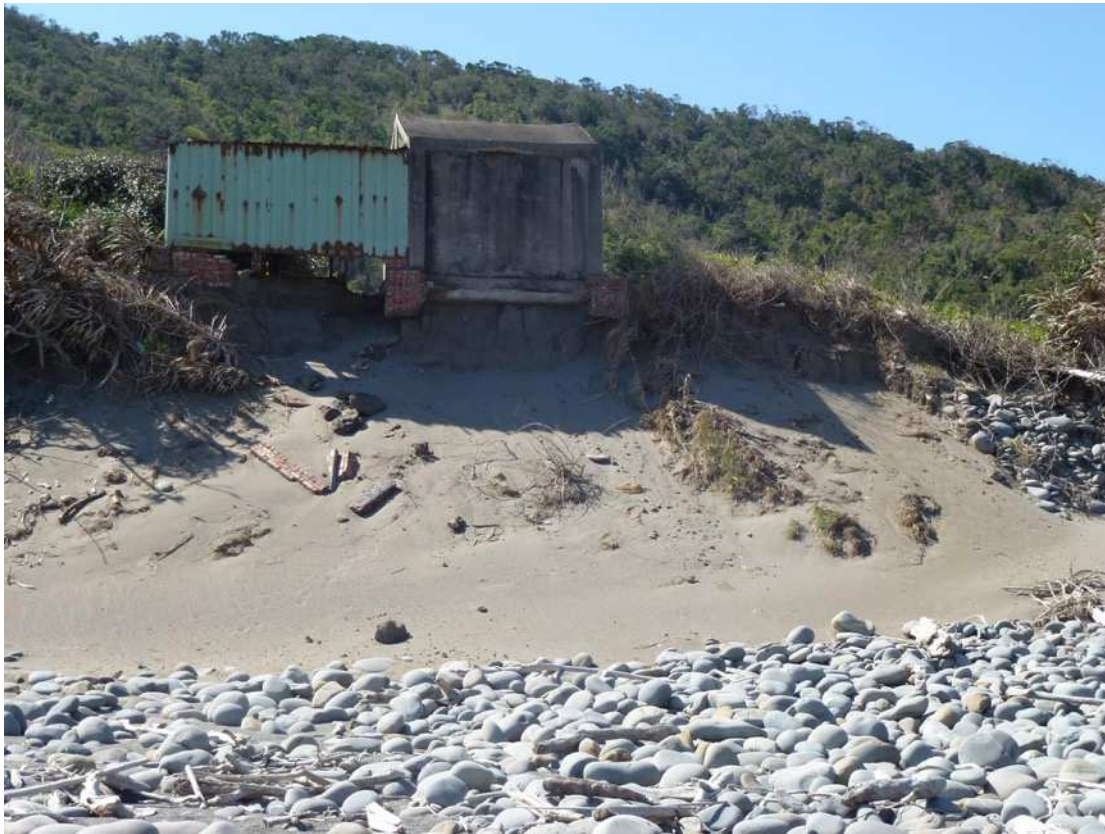
Figure 1 The rising sea level and the shaky house foundations show the villagers' anxiety and the crisis of survival.
