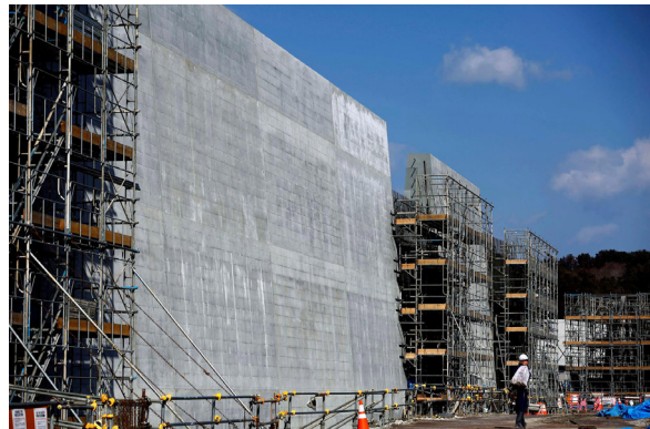
Figure 16. A large sea wall being constructed. Photo by Kim Kyung-Hoon/Reuters (Kyung-Hoon 2018b).
