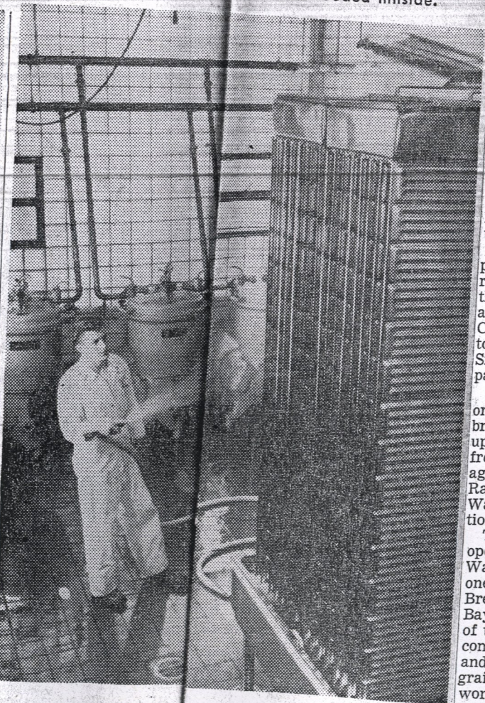
COOLING THE BEER: Beer hot from the brew kettles at the Rainier Brewery is cooled before it can be stored in aging cellars. The cooler is laced with pipes carrying ice-cold water. The pipes cool the beer to 48 degrees.
