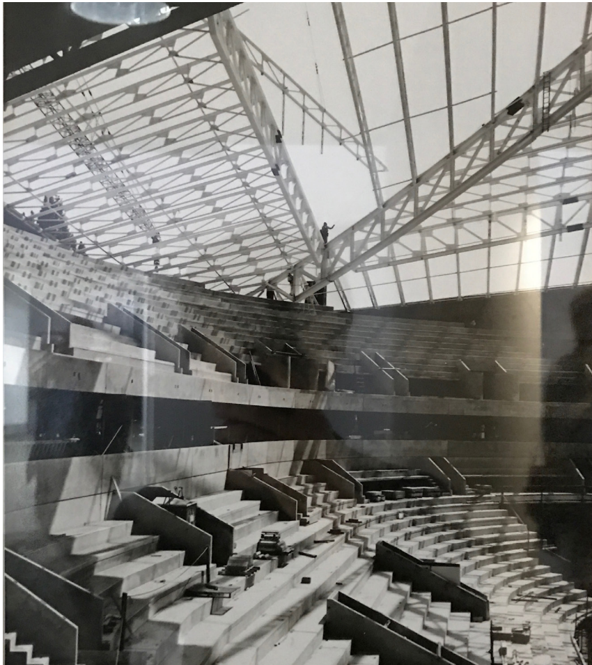
KeyArena renovation photo taken by Lara Swimmer during the installation of the roof structure.
