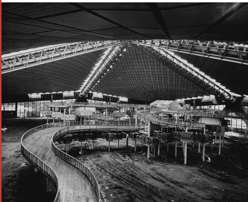
Interior scene under the majestic roof, the ramp and supporting structure of what will be the "World of Tomorrow." From a Seattle Times press shot by Paul V. Thomas for Jan. 3, 1962.
