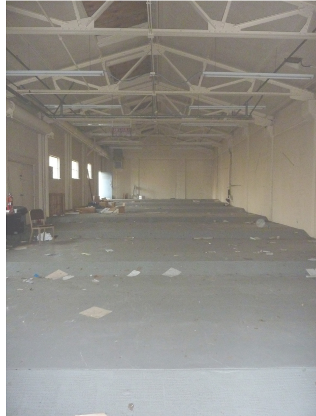
Figure 36: The north building's sloped and flat floor condition to accommodate the sloped topography of 34th Street, 2013.
