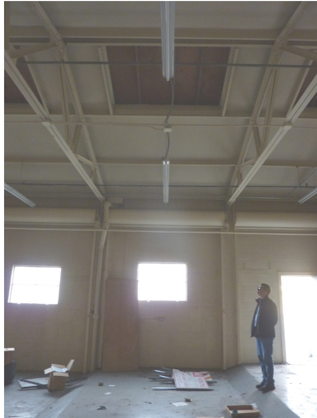
Figure 35: The north building's roll-up garage doors and unique floor condition, 2013.
