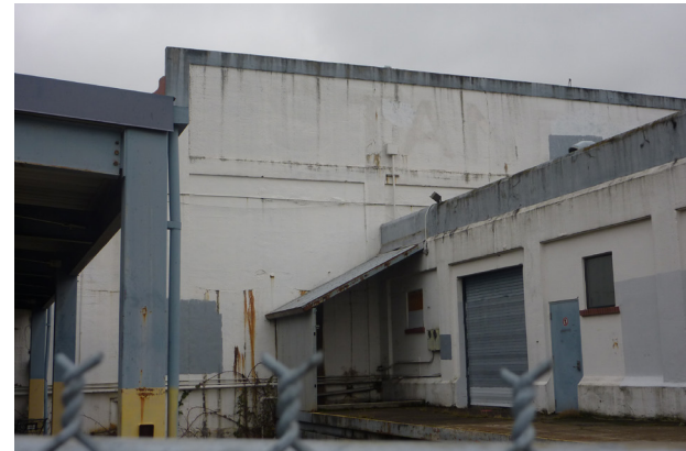
Figure 46: The containment wall facade facing Lake Union still shows evidence of the original "Standard Oil" sign. 2014.
