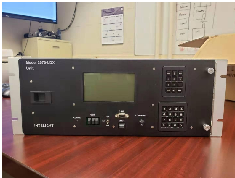
Figure 4: INTELIGHT 2070-LDX controller
