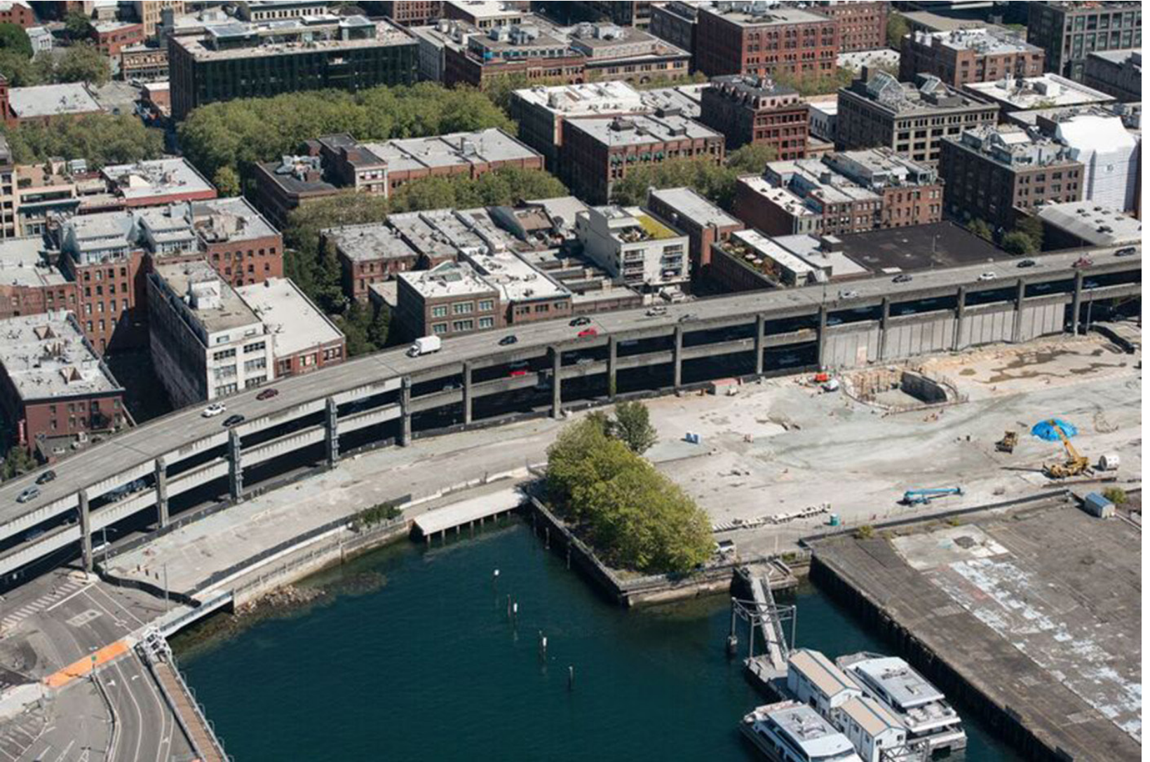
Figure 4.12 Photograph of partial Pier 48 and the Alaskan Way Viaduct near Occidental Square.
