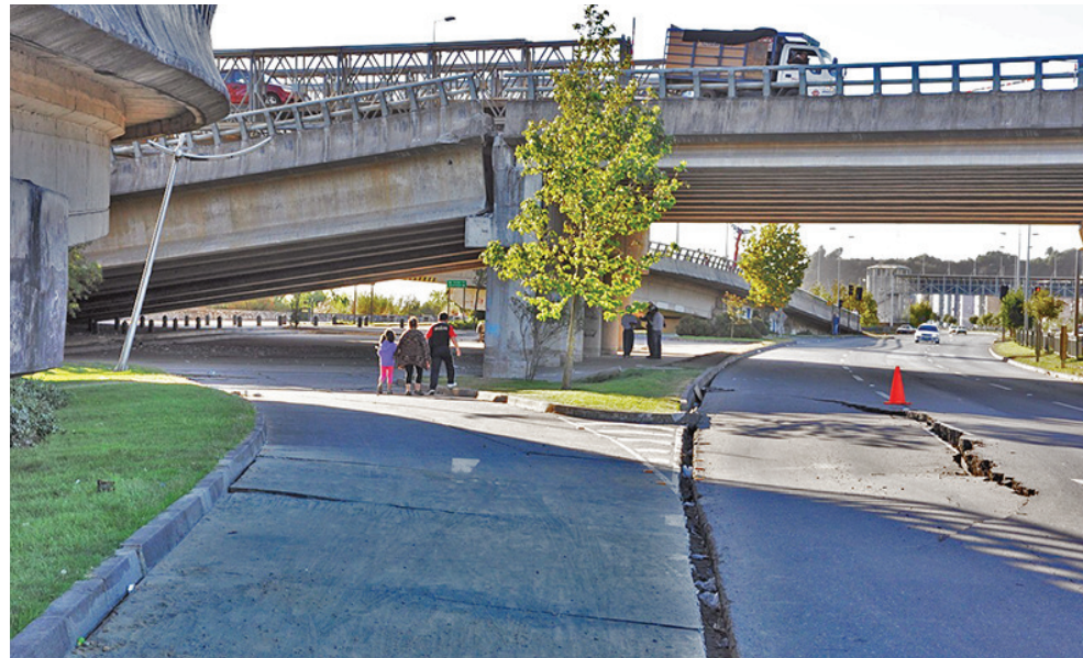
Ground Cracks Extending to the Street
