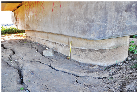
Settlement at Entrance Piers
