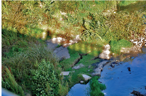
Ground Cracks at the River Bank
