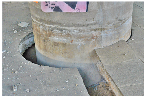
Separation of the Pavement
