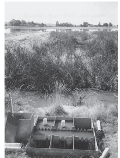
After undergoing primary treatment in a partially aerated pond, wastewater flows to a “splitter box” with V-notches that control the loading rates into four wetland cells.
