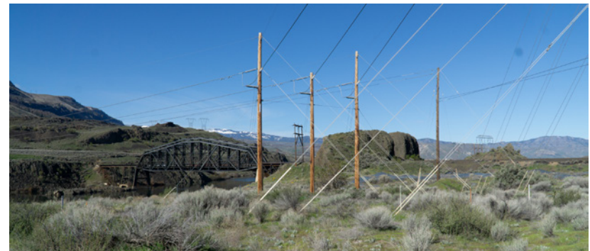
Figure 4.15: Power lines in front of the railroad bridge. April 2019.
