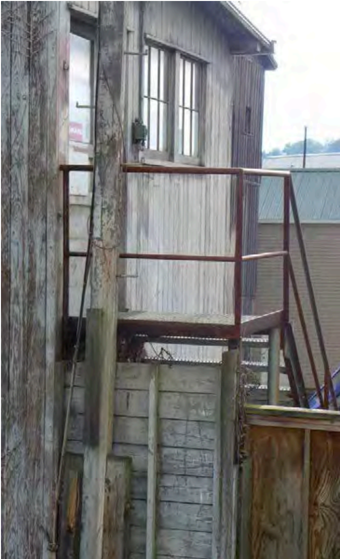
Image 3: Side stair for one of the early wooden structures at the Lake Union Dry Docks.
