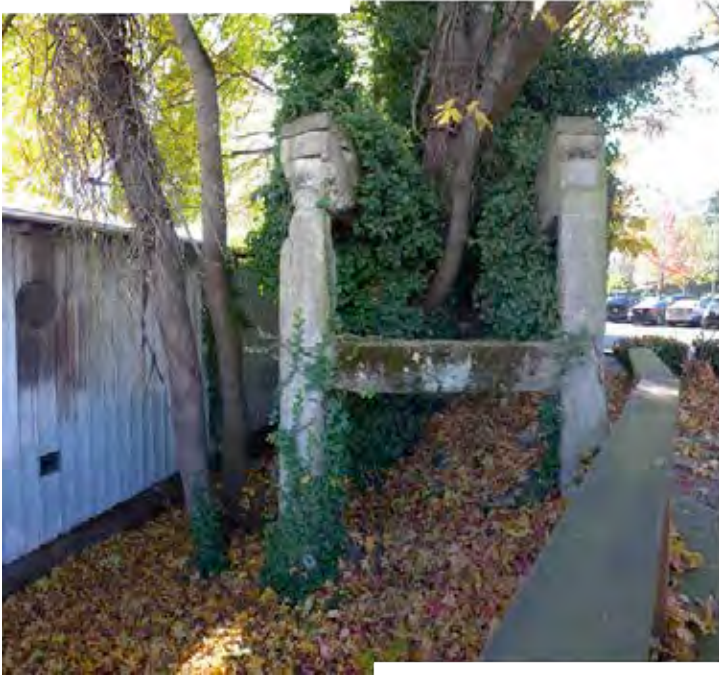
Image 20: English ivy scales the remnants of a concrete trestle that sits beside an actively used parking lot.
