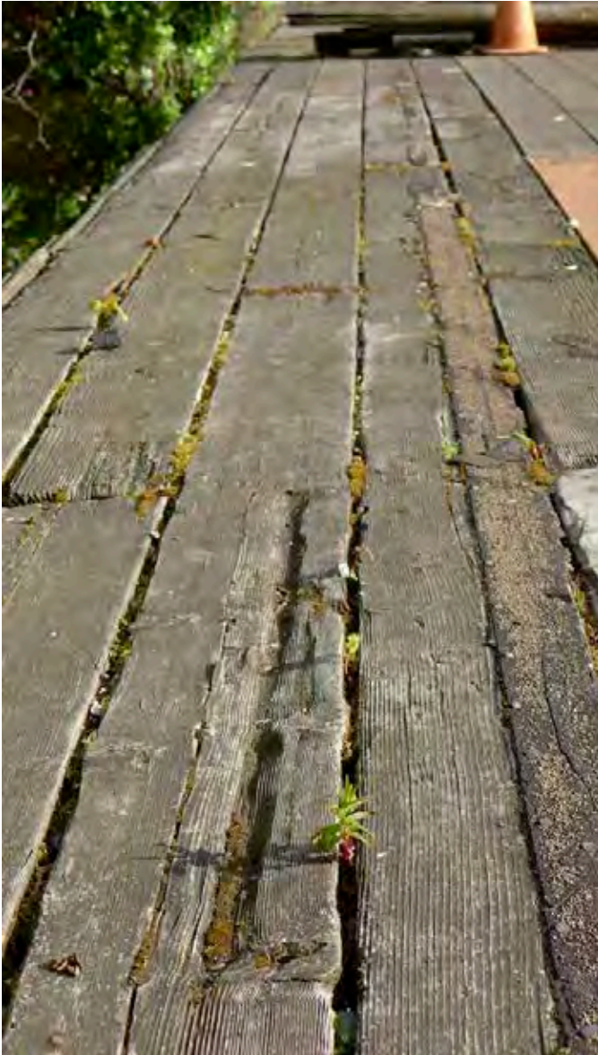
Image 5: Moss and other vegetation grow upon and between the floorboards of the wooden walkways near the Dry Docks.
