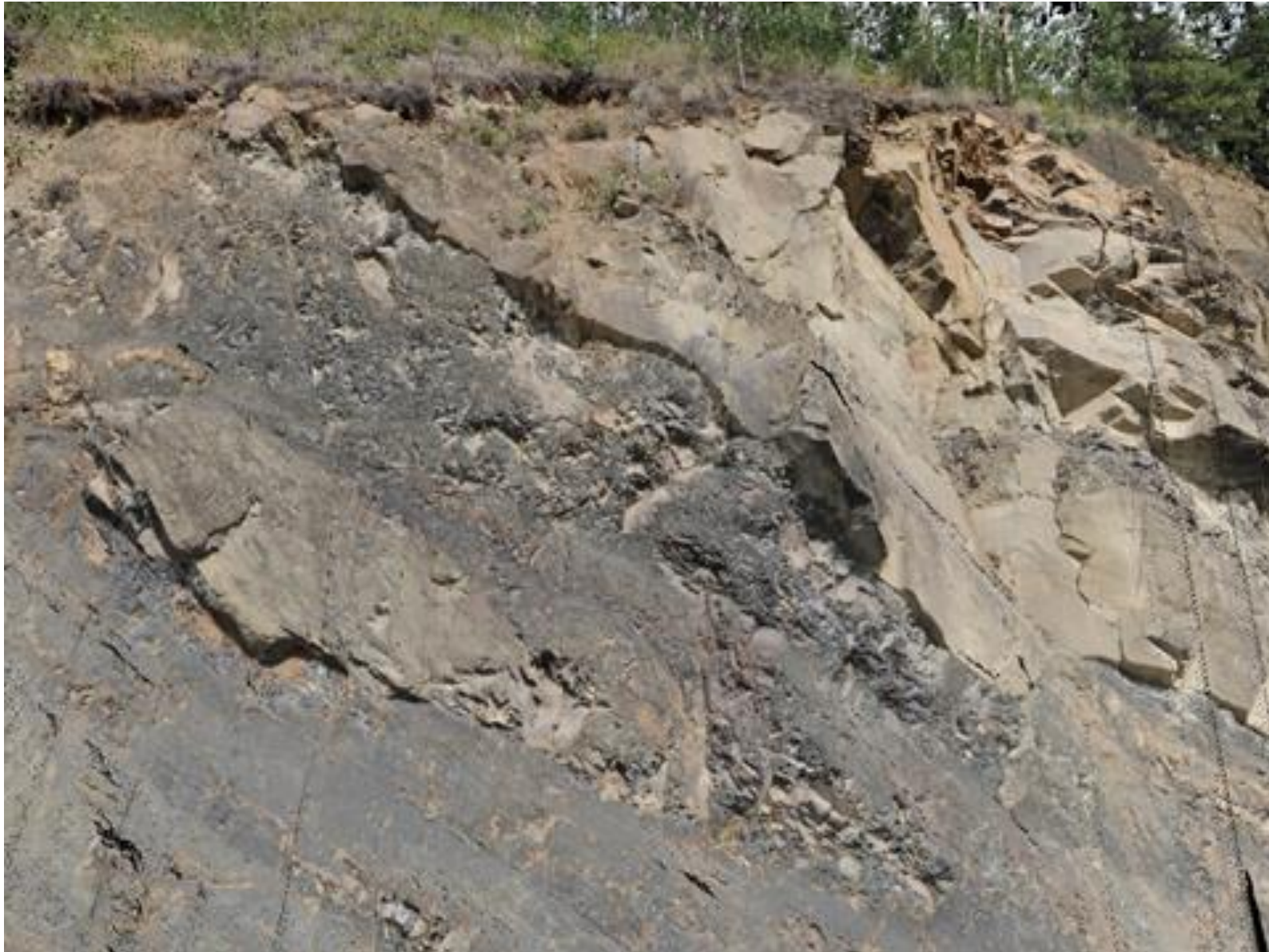
Figure 5.4: Example of 2013 lidar scan from an area along Parks Highway in an area that has highly unstable rocks.
