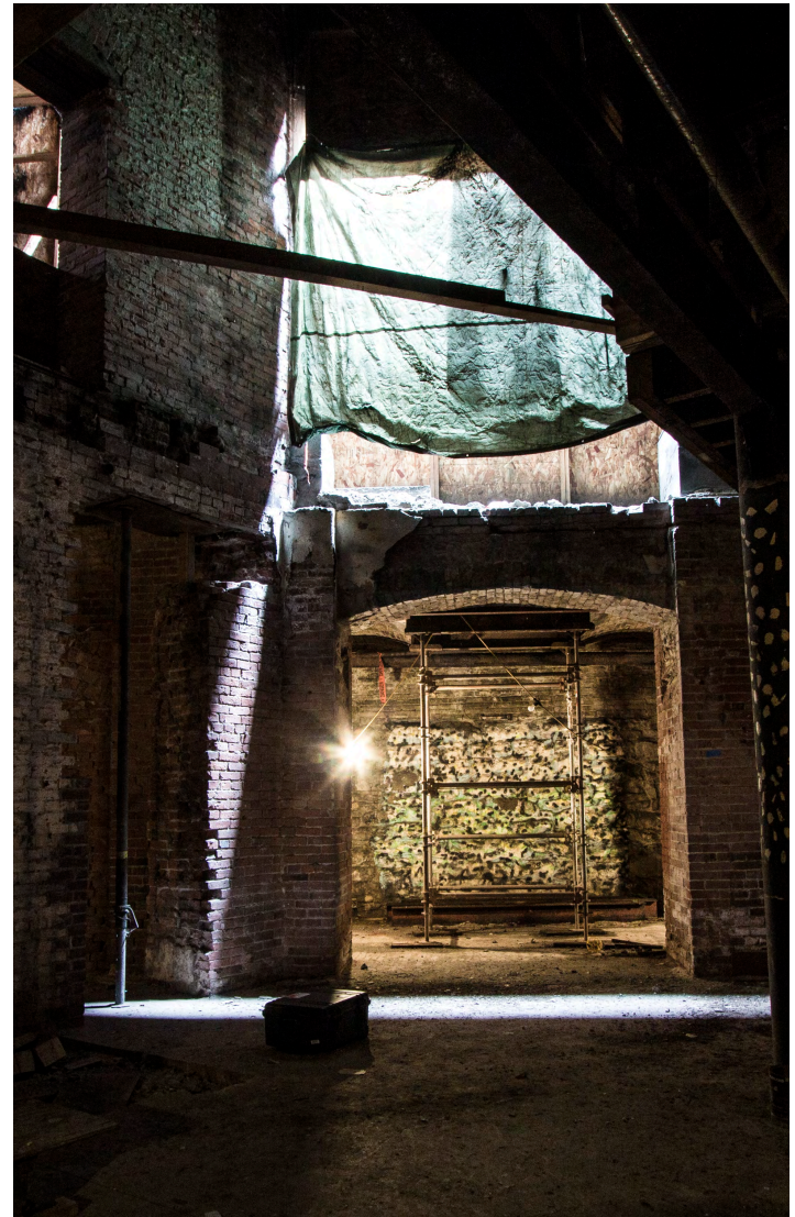
Fig. 43 - Fire Witness Mark
