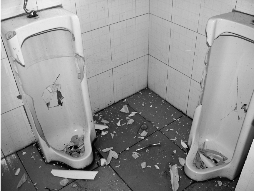
FIGURE 5.2. Urinals in the public toilet at viewpoint number 1, in Ping'an, were smashed as a retaliatory act against changes proposed by the management company (2007). Photo by the author.
