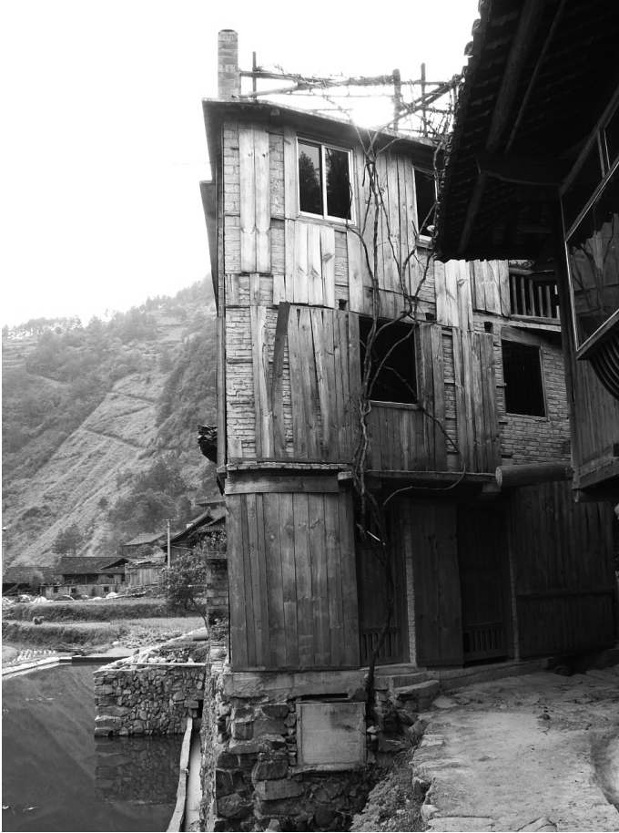
FIGURE 4.3. Wooden planks were used to cover up brick and concrete walls in Upper Jidao, but over time they warped and fell off (2006). Photo by the author.
