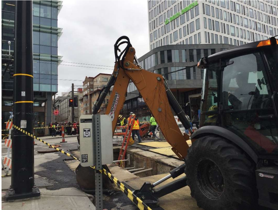
Figure 19: Construction and demonstration at Fairview Ave N and Republican St. Picture taken 2/29/2020.
