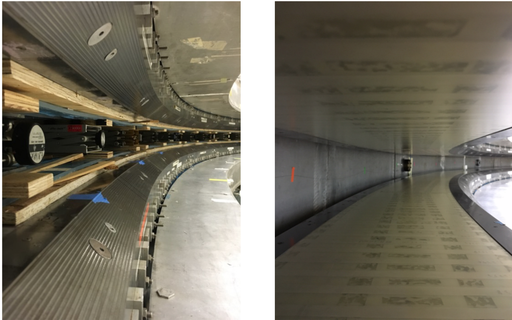
Figure 5.28: The left image shows the full rig used to apply pressure and stabilize the laminations while the epoxy cured over 4 h to 6 h. The rig used a combination of plywood pole covers, curved plastic rails, small metal shims, and wooden wedges to distribute the pressure across all sections of the lamination. The right image shows the finalized laminations affixed to the pole surfaces.
