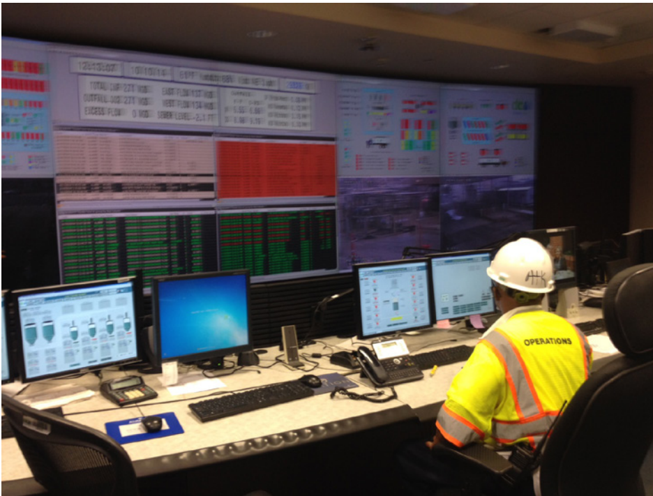
Fig 4: Control Center at Blue Plains Wastewater Treatment Plant, Washington DC.
