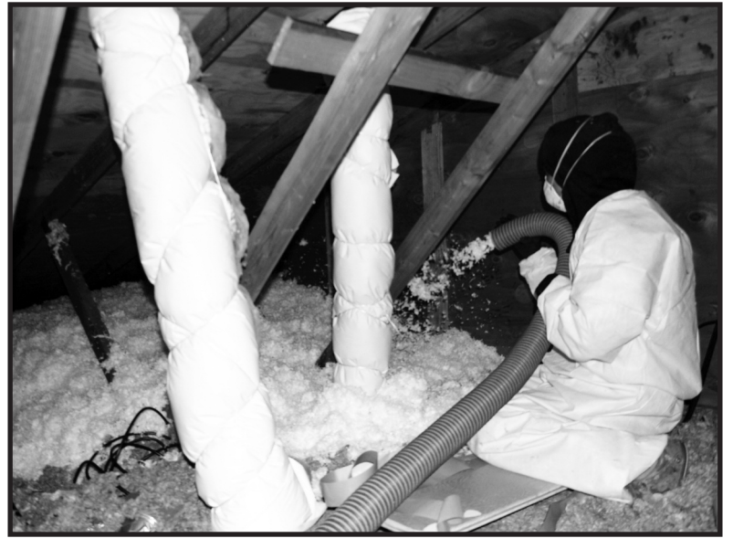
Rochelle Sadler, a member of Laborers Local 296, blows insulation in the attic of a 1986 home in Portland’s St. Johns neighborhood. She is one of 10 full-time employees at Abacus Energy Solutions. The homeowners — Oregon AFSCME lobbyist Eva Rippetateau and her husband, AFSCME international field coordinator Andy Chavira — chose Abacus because it’s a union shop. Chavira said $4,500 of blown fiberglass attic insulation, air sealing, and HVAC improvements will cut their energy bill — and make a couple of chilly rooms more comfortable.
