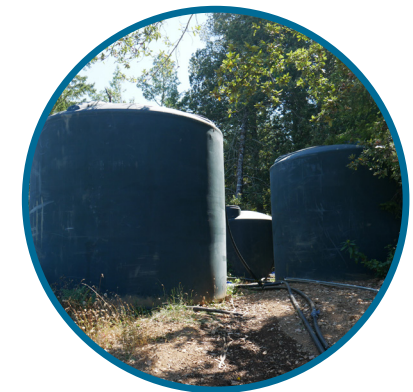
F. Irrigation Tanks
