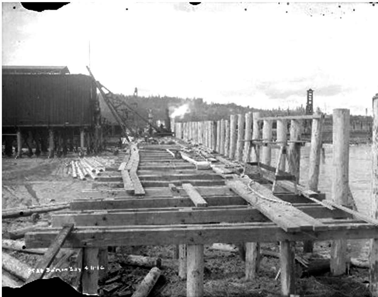
Photo 5.6: Shoreline armoring during the construction of Ballard's Fisherman's Terminal in Salmon Bay, April 11, 1914. (Credit: Seattle Municipal Archives).
