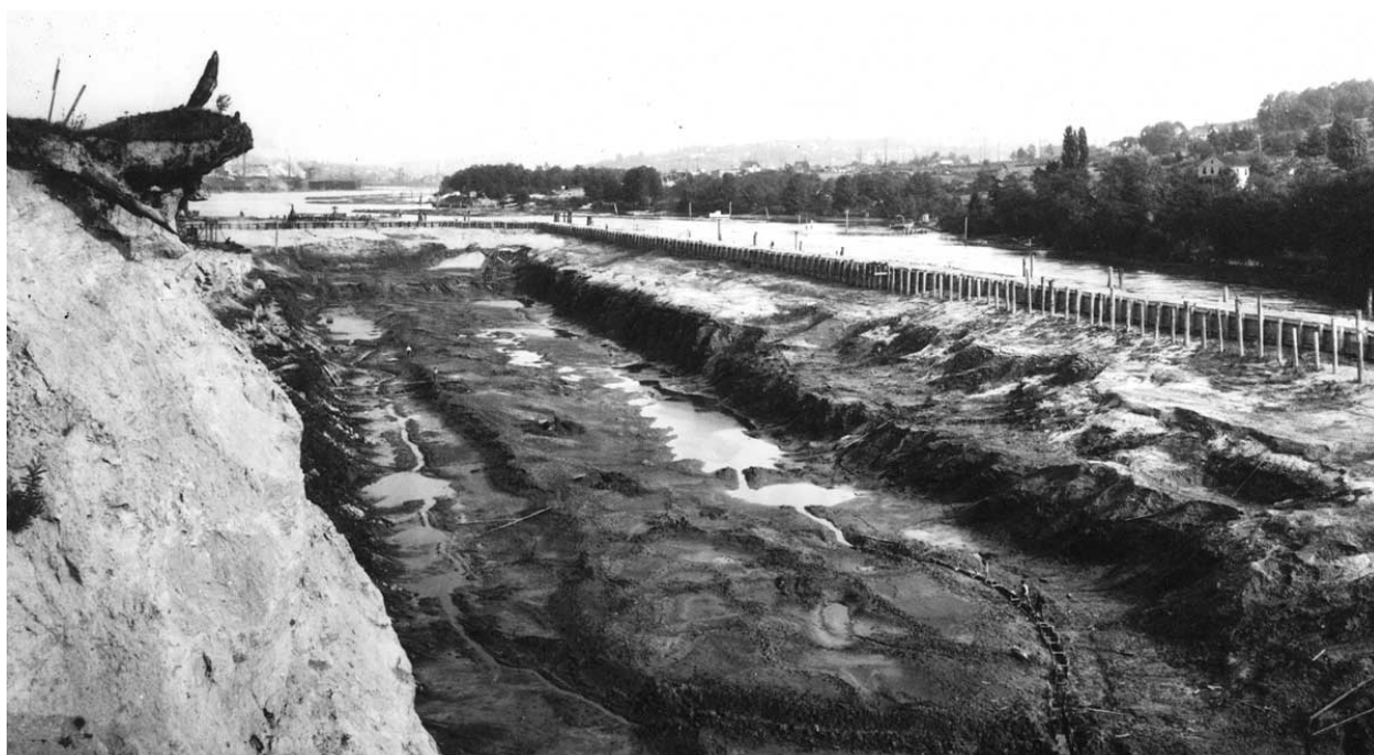
Photo 5.4: The Ballard locks under construction in 1912. View looking east toward Magnolia and Salmon Bay (Credit: US Army Corps of Engineers).
