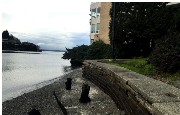
Photo 6.4: Armored shoreline at the NW 57th St street end site in Ballard. (Credit: photo by Rhys van Bommel).
