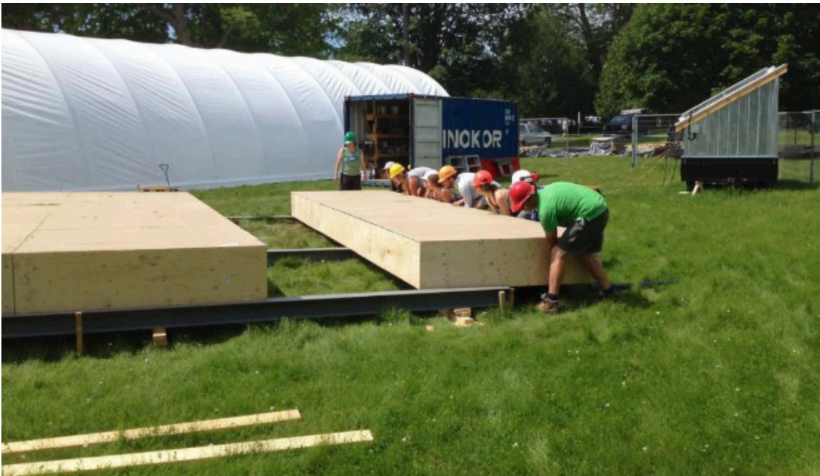
Figure 45. Assembling the floor panels: Sliding the floor panels onto the foundation beams. Endeavour Center and Ryerson University, 2017.
