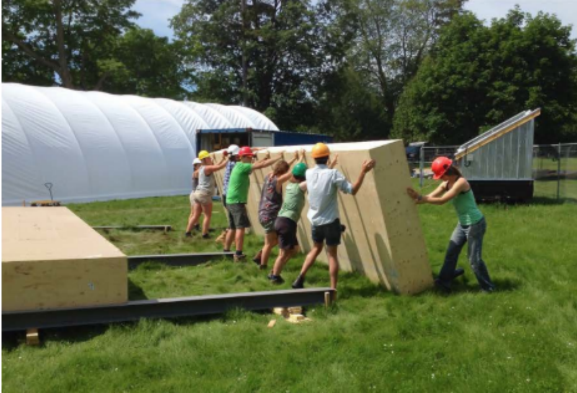
Figure 44. Moving the floor panels from the tent to the foundation by manually using rollers and the power of the whole team. Endeavour Center and Ryerson University, 2017.
