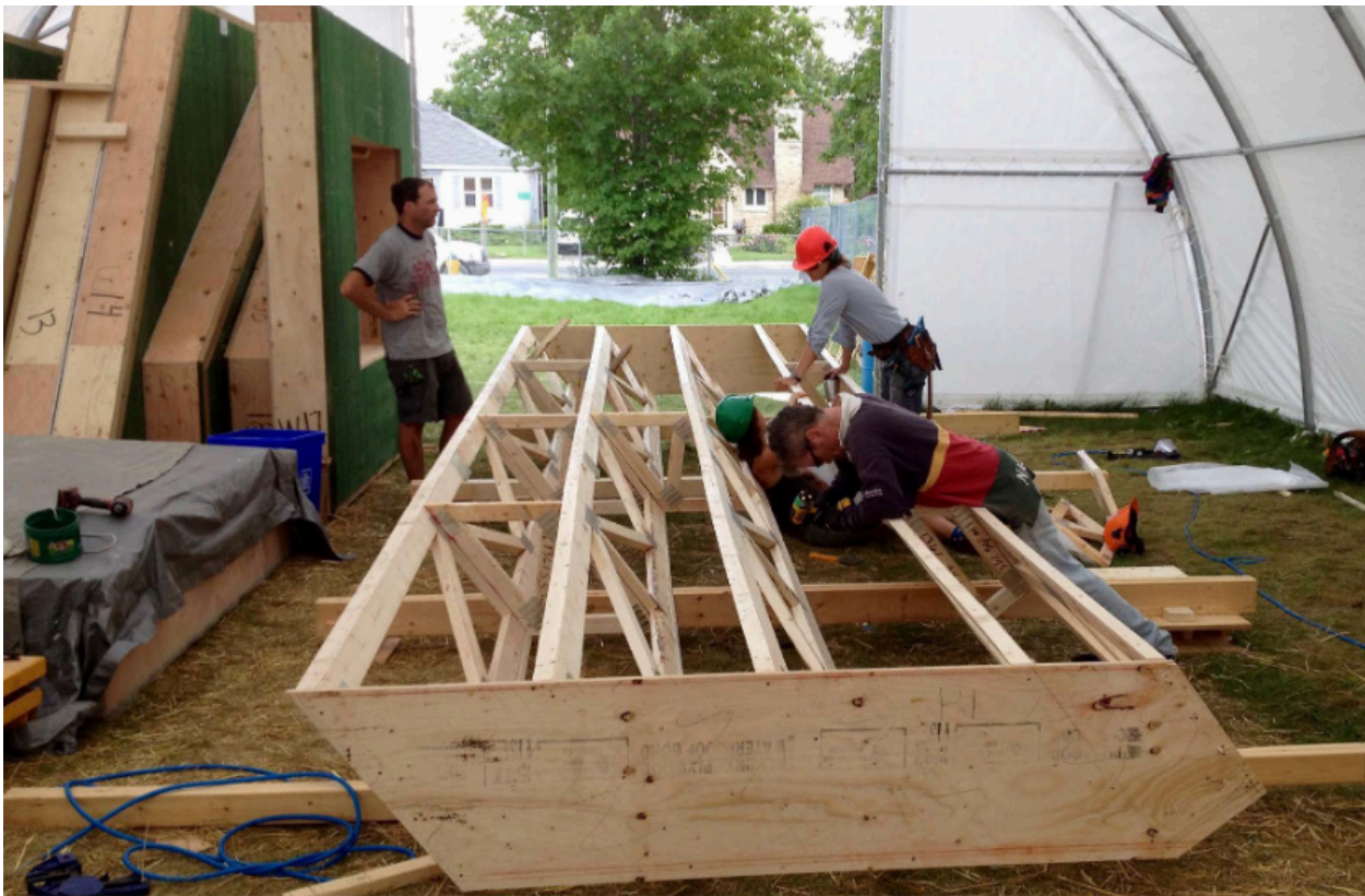
Figure 41. Assembly of angled roof panels inside the "Flying Factory" workspace. Endeavour Center and Ryerson University, 2017.
