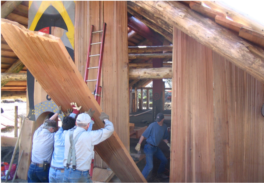
Figure 22. Installing vertical wall planks at the Cathlapotle Plankhouse in Ridgefield, Washington. Advisory Council on Historic Preservation, n.d.
