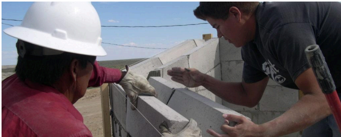
Figure 16. Nageezi House was built by volunteer student labor and the Navajo Housing Authority construction crew, 2005.
