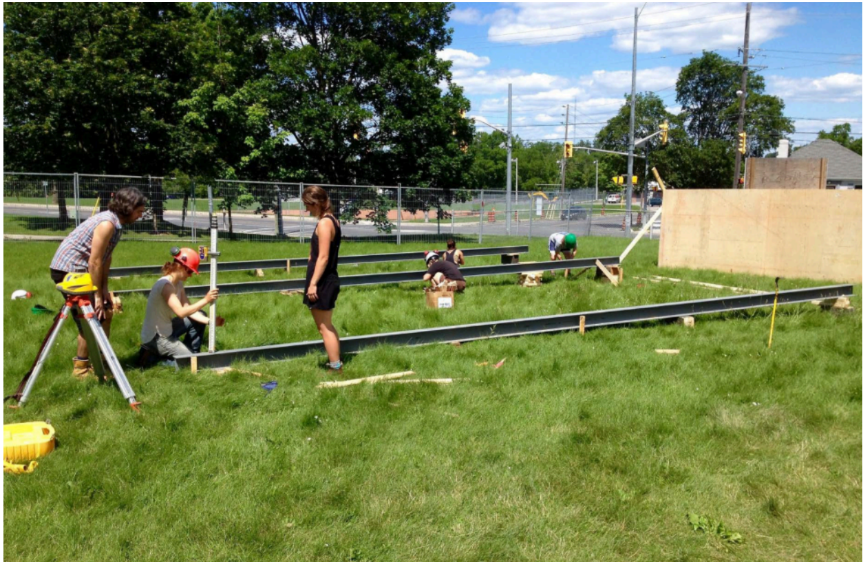
Figure 43. A temporary platform foundation for the building using steel beams. Endeavour Center and Ryerson University, 2017.
