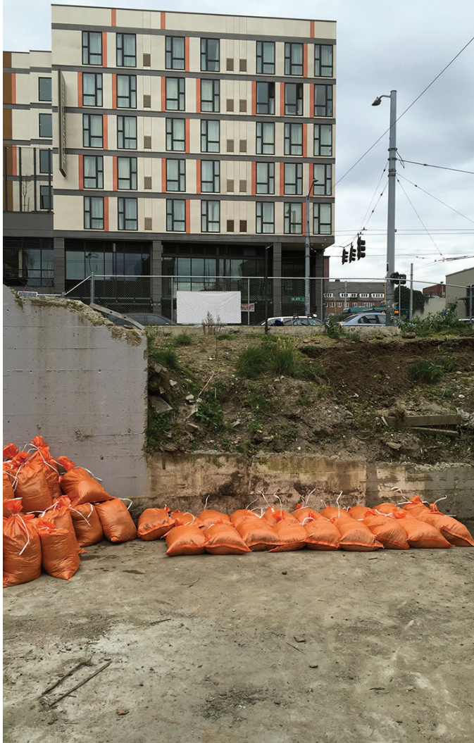
Foundation ruins during initial site clean-up. Sand bags containing dirt and rubble were later used to retain the excavated grade pictured here.
