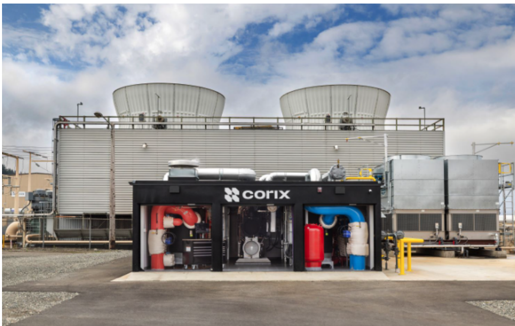
Figure 4.2 Waterfront district energy central plant (Corix, 2023)
