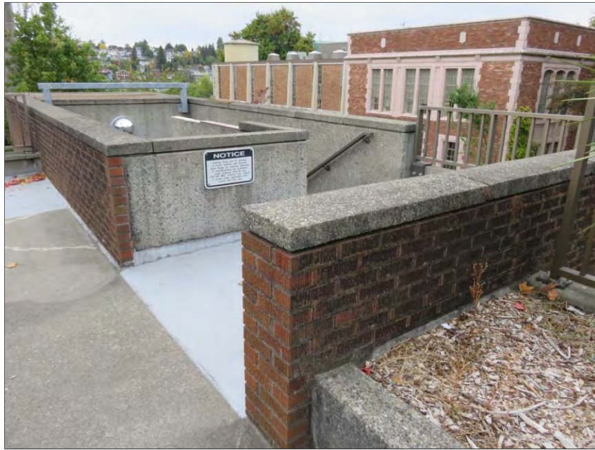
Figure 8-79. Brick trim and concrete stairs at southwest corner of South Campus Parking Garage, view southwest.
