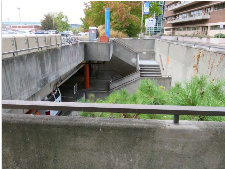
Figure 8-80. Northern stairwell along north wall of South Campus Parking Garage, view west.
