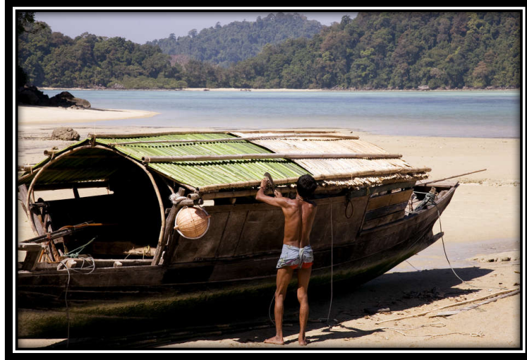
Figure 4- 4. A Moken man named Pe Tat uses palm leaves to make a new roof for his family’s kabang
