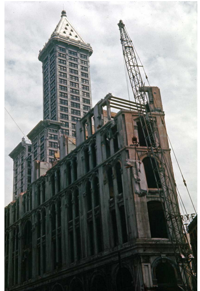
Figure 9. The Seattle Hotel, successor to the Occidental Hotel destroyed in the 1889 fire, being demolished in 1961. The "Sinking Ship" parking garage was built in its place and its destruction was a key event in establishing the Pioneer Square Preservation District.
