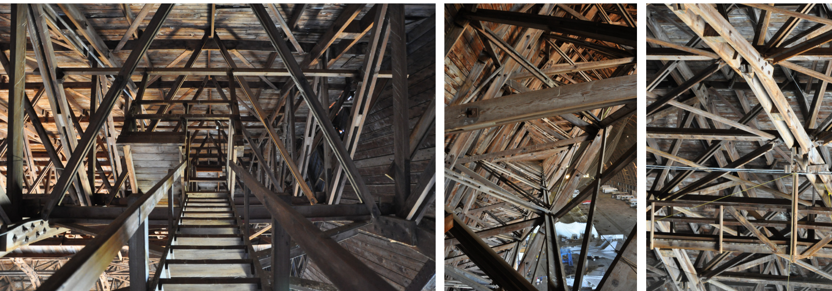
view up access ladder view down length of hangar upper level catwalk
