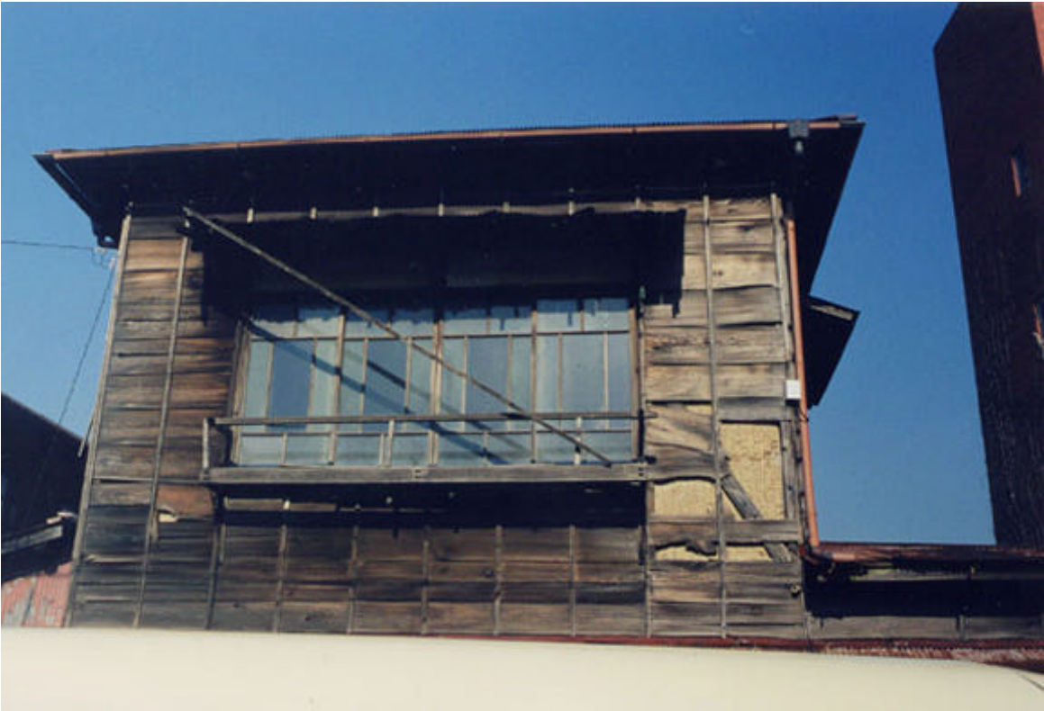
Figure 34. Poor quality windows and construction practices contributed to moisture infiltration around and through wood windows.
