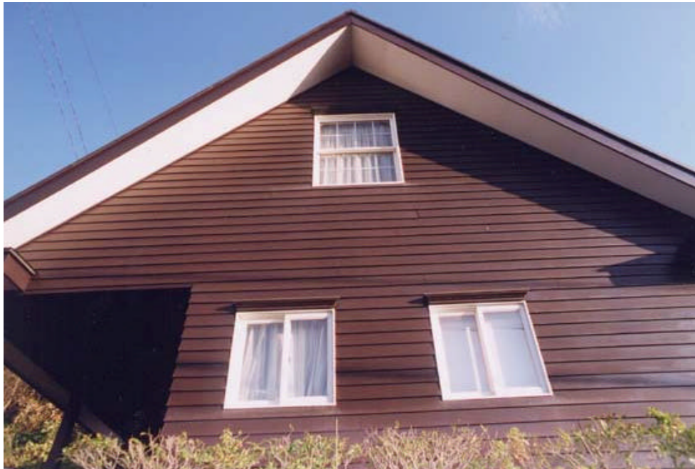
Figure 39. Small window overhangs on this older wooden house are an effective way to deflect rain water away from the window opening.
