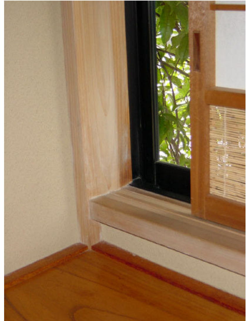
Figure 50. Detailed view of a shiiki (bottom track) for a sliding shoji screen illustrating how it slides under the casing return.
