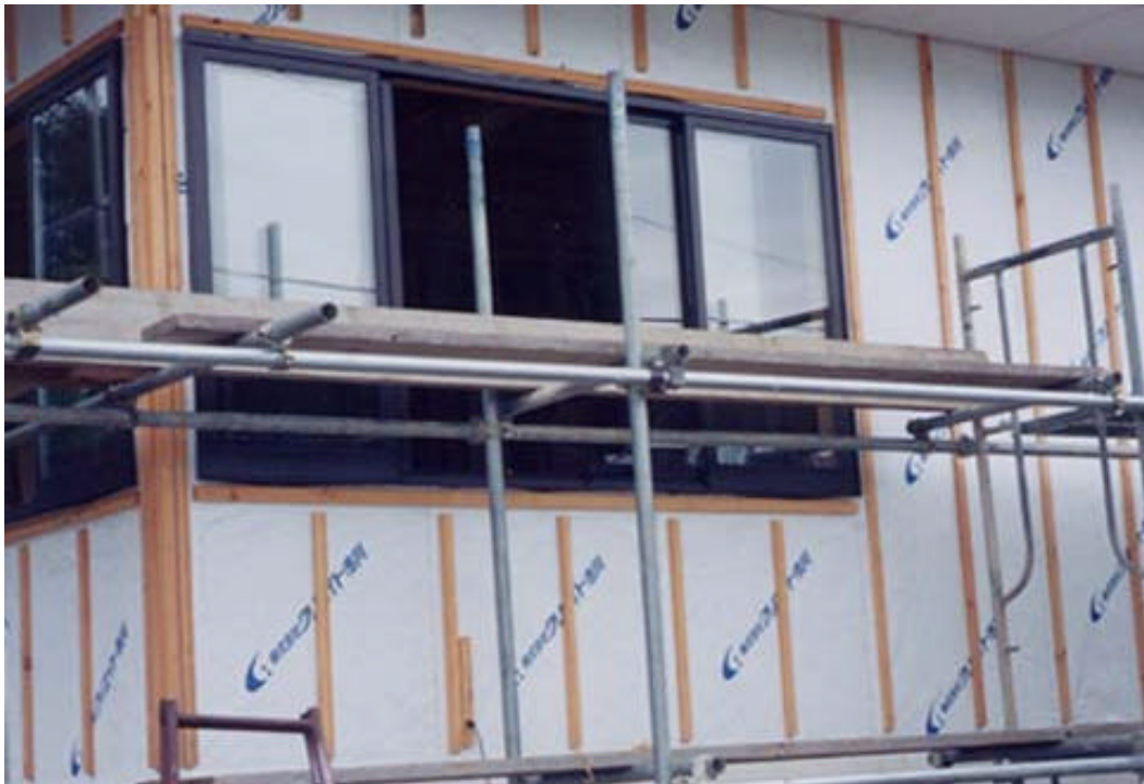
Figure 44. Windows are installed flush onto the dobuchi strips, thereby necessitating the use of a wider casing for the interior trim.
