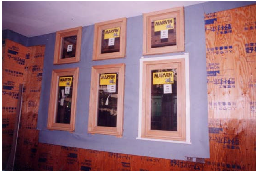
Figure 42. Even in protected areas of the house, using waterproof tape around windows will help prevent moisture related problems.
