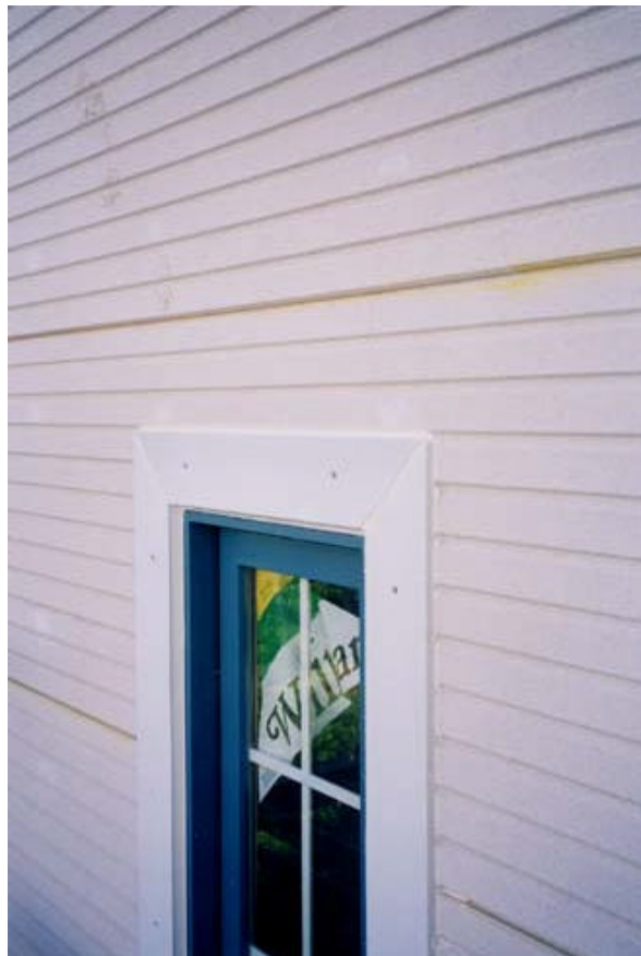
Figure 41. Rain flowing down the exterior wall can penetrate this unprotected window opening and penetrate into the wall cavity as a result of hydrostatic pressure.
