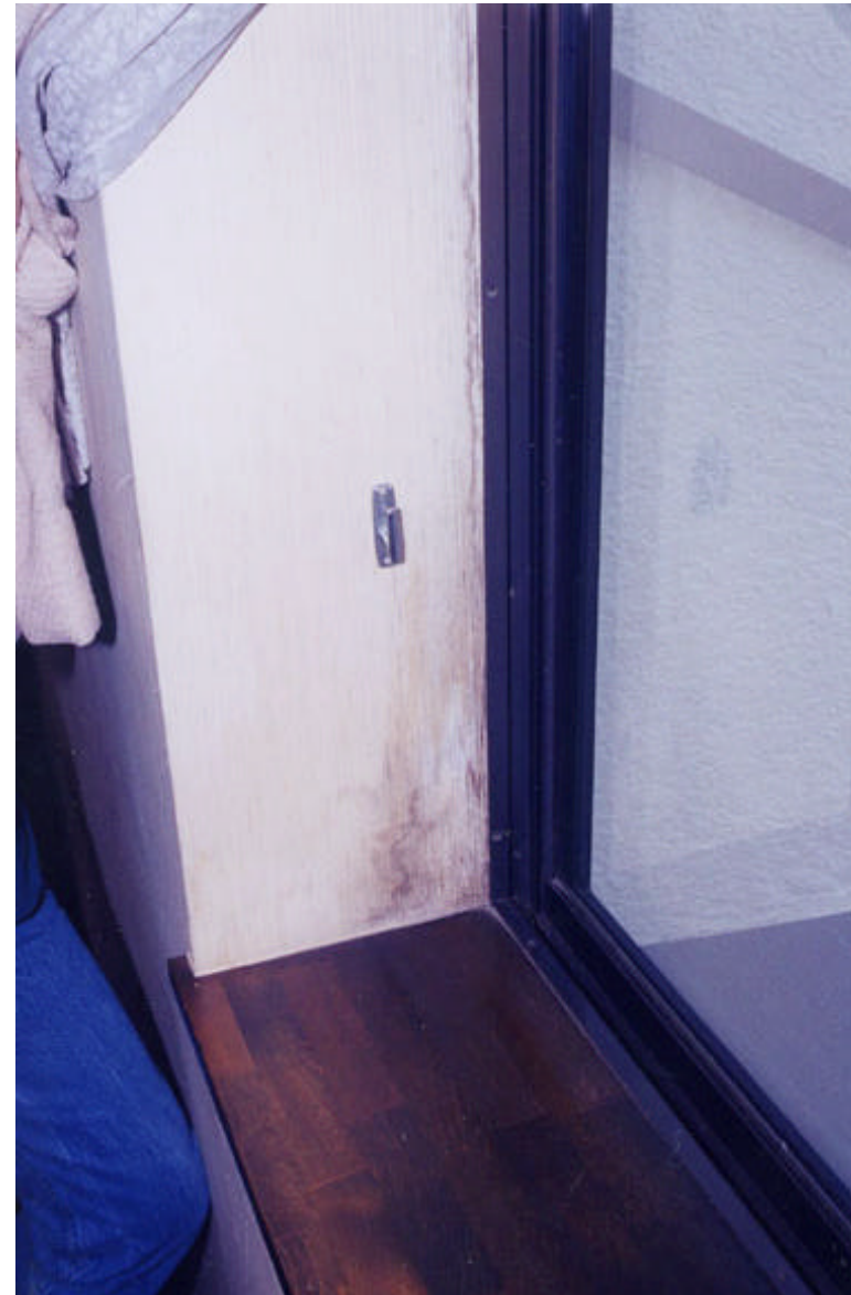
Figure 6. Mold and staining is caused by condensation and water infiltration through aluminum windows.
