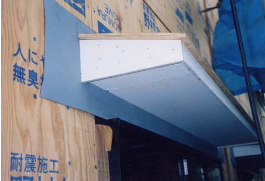
Figure 40. Some home builders build small accent roofs to protect windows from water flowing down the side of the wall.
