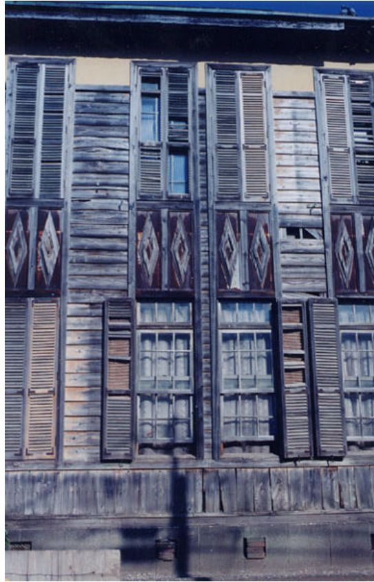
Figure 35. While traditional window designs were interesting poor quality adversely affected performance in Japan's hot, humid and wet climate.
