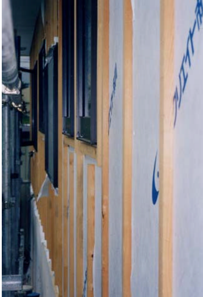
Figure 45. These windows were installed flush with the wall and the dobuchi strips were added. This is not a recommended installation technique and can result in the exterior wall surface being flush with the window surface as shown in Figure 34.
