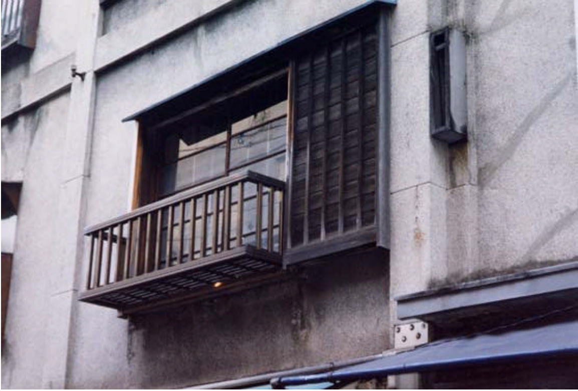
Figure 33. Traditional wood windows were often poor quality and poorly maintained.
