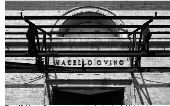
Figure92: Macello Ovino door and overhead rail system in Mattatoio (sheep slaughter).
