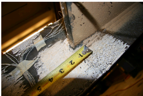
a. 3/4 in. weld crack (WB1) at -1.5% drift
