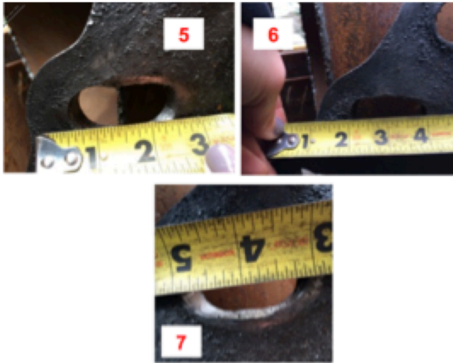
Figure 5.57 - Bolt Hole Elongation in NE Gusset Plate
