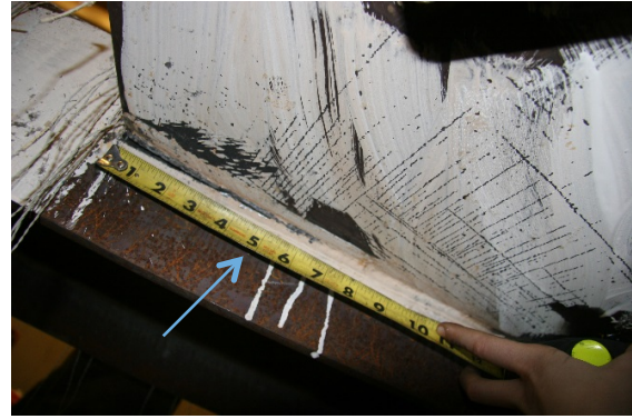
b. Moderate Weld Tearing , WB2
