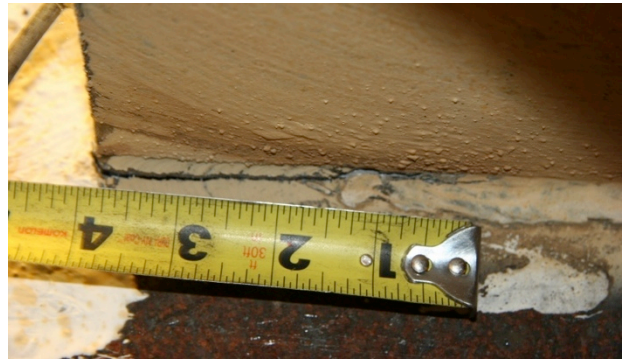
b. 4 in. (bottom) & 1 in. (top) weld crack at -1.6% drift
