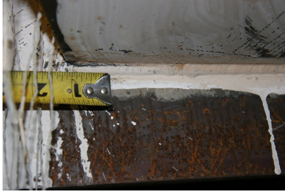
a. Initial Weld Tearing, WB1
