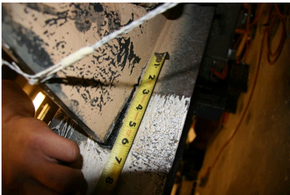
e. 6.5 in. weld crack (bottom) at -2.9% drift
