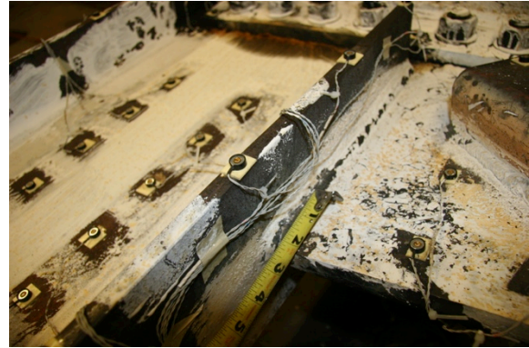
d. 2.25 in. weld crack (top) at -2.7% drift
