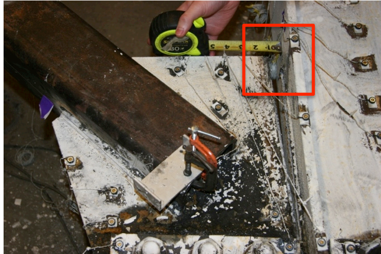
Figure 5.45 - 1 in. Gap Between NE Gusset Plate and Beam at +0.88% Drift
