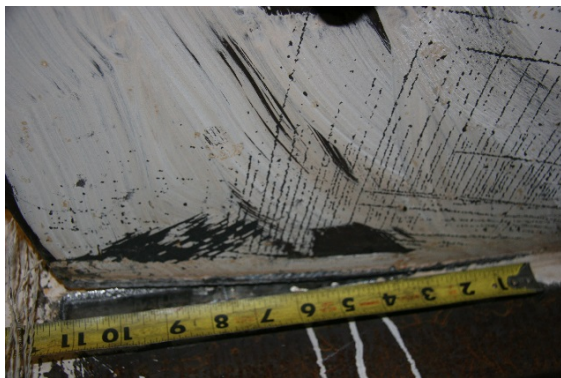
c. Severe Weld Tearing, WB3
