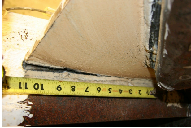
d. 11 in. (bottom) & 8.5 in. (top) weld crack at -2.1% drift (first cycle)
