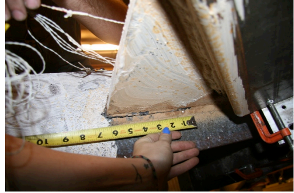
d. 6 in. Weld Crack (WB2) at Beam to Gusset Plate
