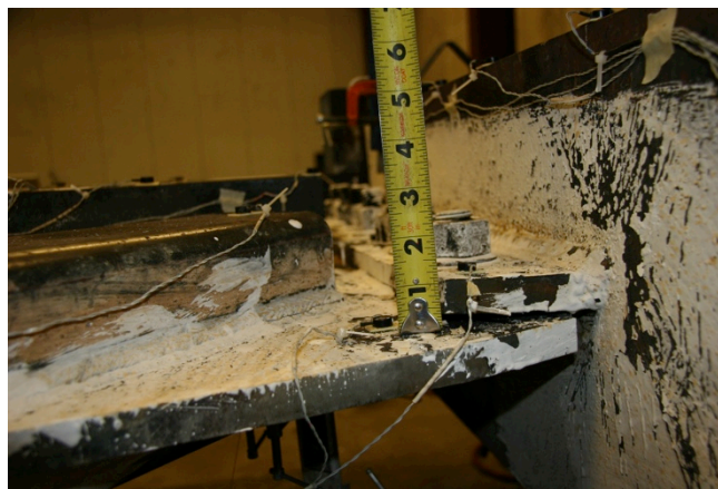
Figure 5.16 - Gap Between Shear Plate and Gusset Plate in NE Corner
