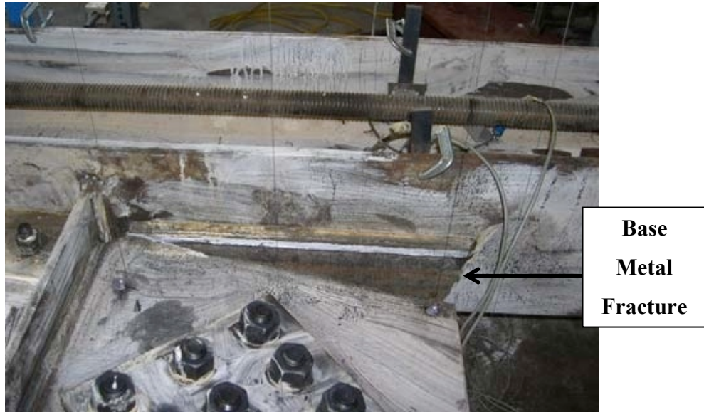
Figure 2.8 - NE Column Connection Base Metal Fracture at -2.66% Drift (modified from Kotulka, 2007)
