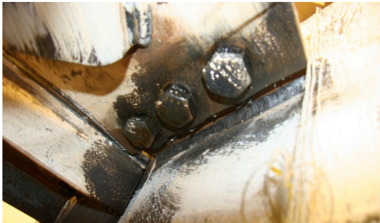
Figure 5.46 - Bolt Hole Elongation in the Gusset Plate in the NE Corner
