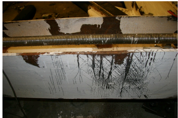
b. Severe Yielding (Y3) on West Flange
