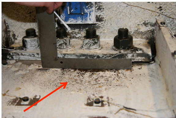
a. Local Buckling of Beam Web NE Corner
