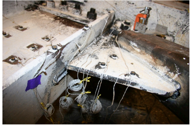
e. Post weld fracture at -3.7% drift
