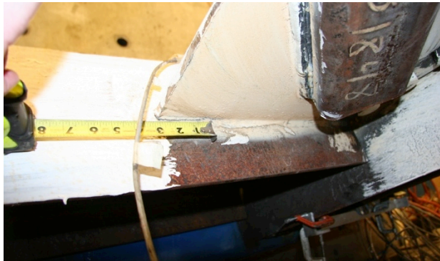
a. 2.75 in. long weld crack at -1.3% drift
