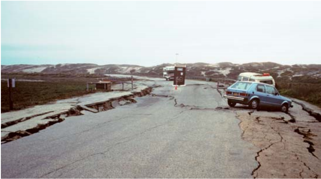
Figure 2.5: Ground failure in Moss Landing, CA, due to lateral spreading, after the 1989 Loma Prieta Earthquake (USGS)
