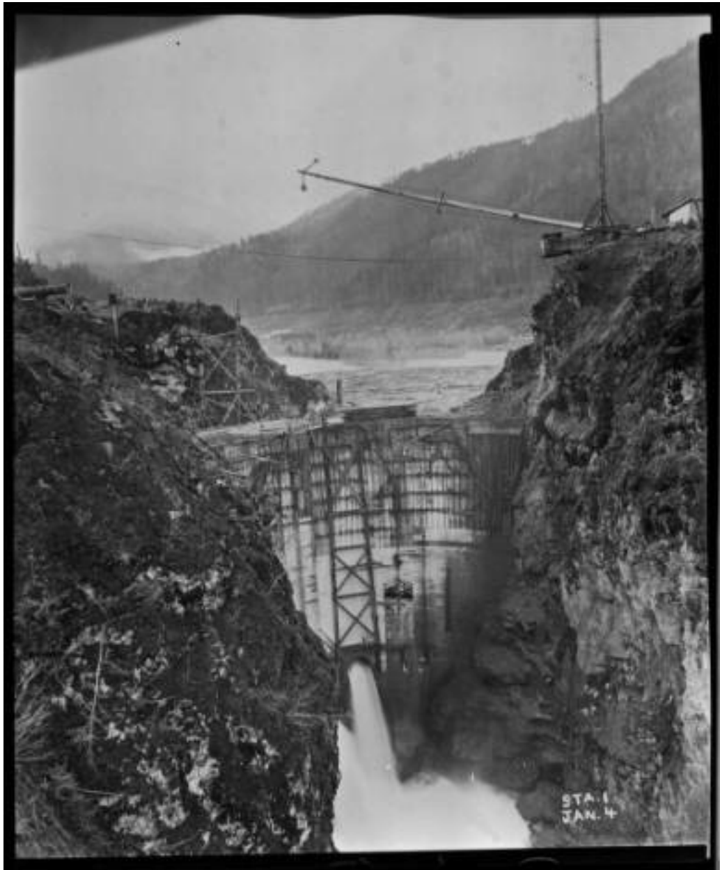
Figure 4. Upper Elwha (Glines Canyon) Dam Under Construction, c.1927, Photograph. Burt Kellogg Collection. Courtesy of the North Olympic Library System, accessed April 5, 2014, http://www.washingtonruralheritage.org/cdm/singleitem/collection/nols/id/93/rec/17 .
