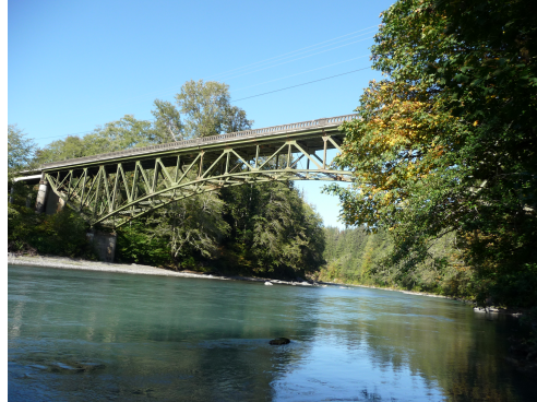
(b) Under-truss and Pratt type bridge which the deck is supported directly by upper chord and the all diagonals are in tension
