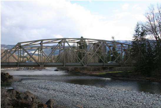
(a) Through-truss and Warren type bridge which the deck is supported directly by lower chord and the diagonals are in tension and compression alternately
