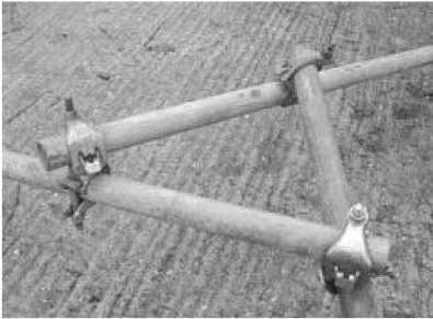
Fig. 2.12: Friction-dependent clamp fittings are highly adaptable to changing geometric demands, but are not well-suited to resisting axial loads.'
