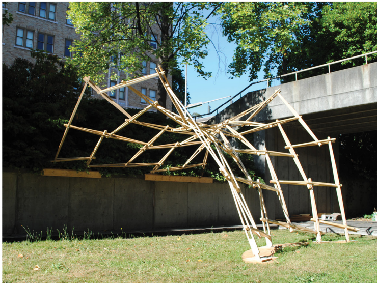
Fig. 5.27: The pavilion's hyperbolic geometry is generated by the interaction of unique beam lengths, and requires no false-work to create curved edges.
