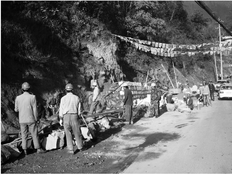
FIG. 4.3. A team of migrant workers from Dali Prefecture constructs retaining walls along the main street of the Gongshan county town (December 2006).
